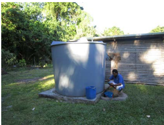
Figure 12 One of the six tanks installed by the CBDAMPIC project. The rainwater-capture shelter, converted into a guesthouse, is in the background.
