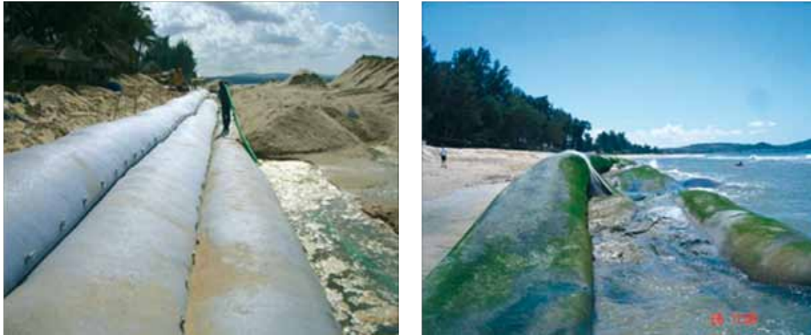
Figure 30: Beach protection project at Doi Duong, Phan Thiet City, Binh Thuan Province by Geotubes (Photos: SIWRR)
