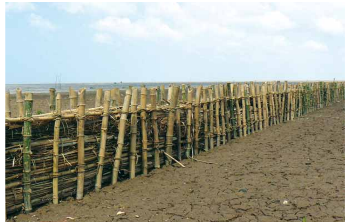
Figure 25: Bamboo breakwater in Vinh Tan Commune in Soc Trang Province (Photo: Albers)
