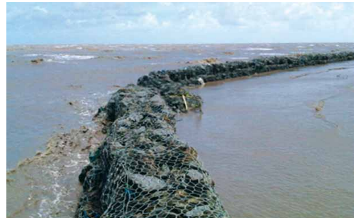
Figure 22: Detached breakwater consisting of gabions at the West Sea coast at Vam Kenh Moi (near Da Bac), Ca Mau Province (Photo: SIWRR)
