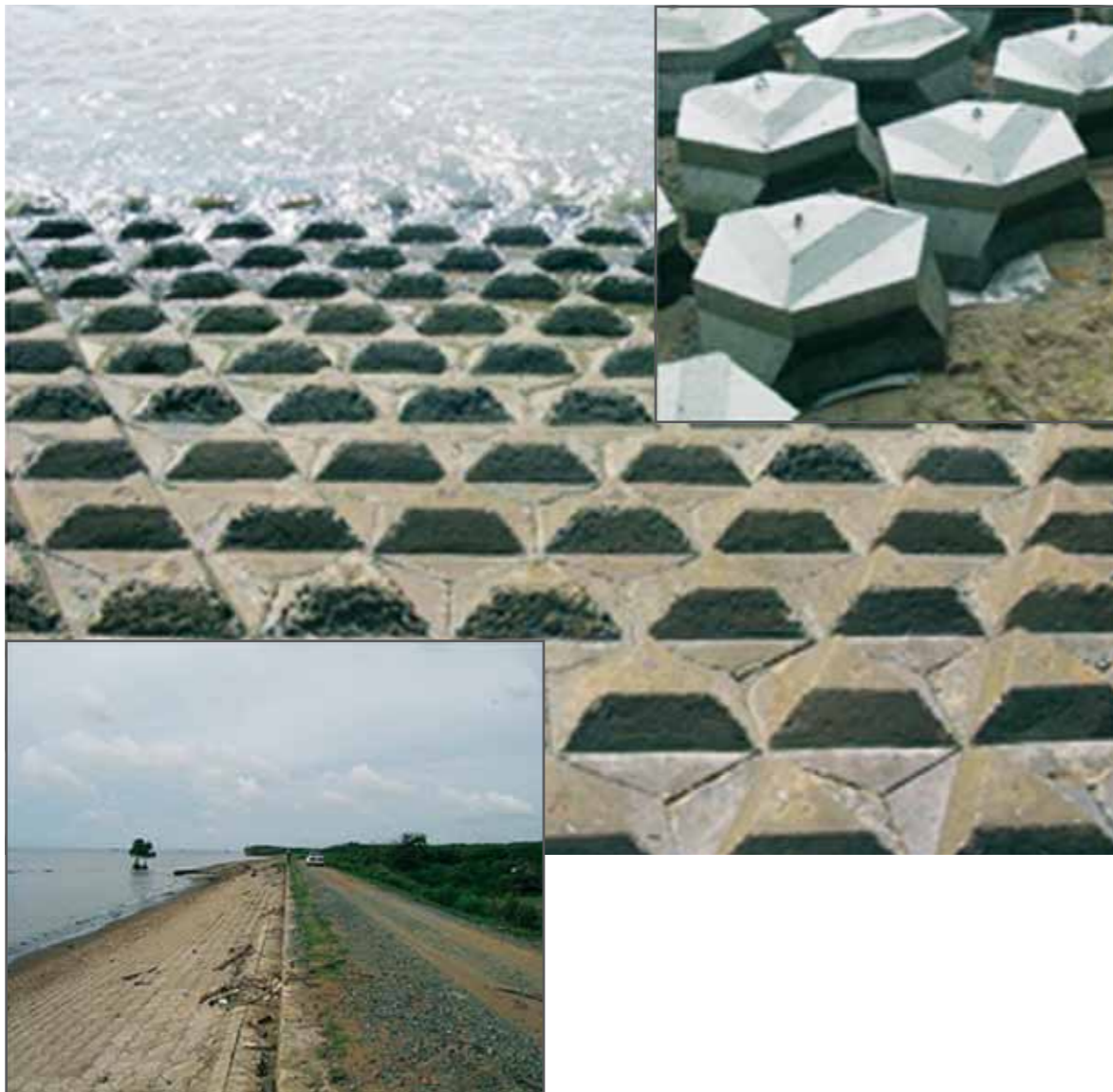
Figure 27: Revetment of concrete blocks on the coast of Go Cong District, Tien Giang Province (Photos: SIWRR)
