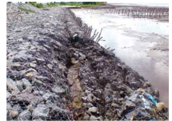
Figure 29: Gabion revetment at a sluice gate in Soc Trang Province (left), damaged gabion revetment in Vinh Tan Commune, Soc Trang Province (right); (Photos: Albers)
