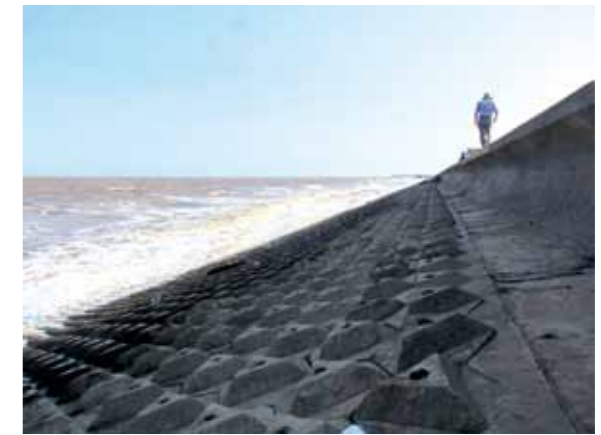
Figure 28: Revetment of concrete blocks combined with a low sea wall at the coast of Tra Vinh Province (Photo: Pham Thuy Duong)
