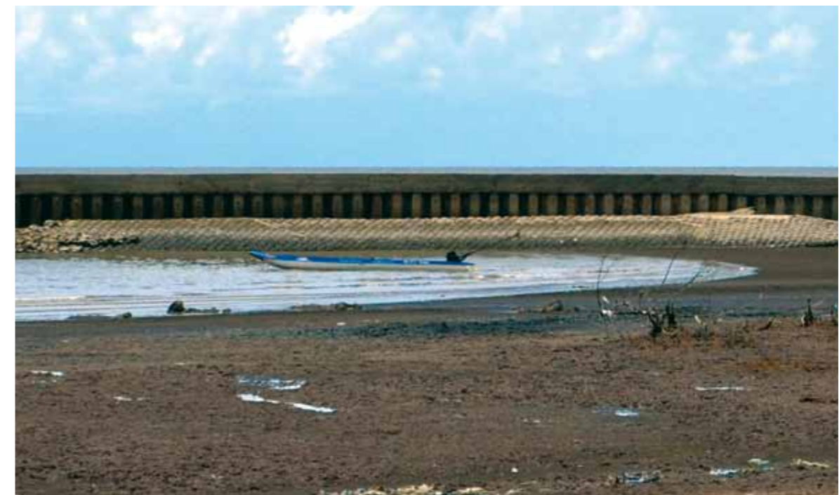
Figure 34: Structure of a seawall at Ganh Hao, Bac Lieu Province (Photo: GIZ Bac Lieu)
