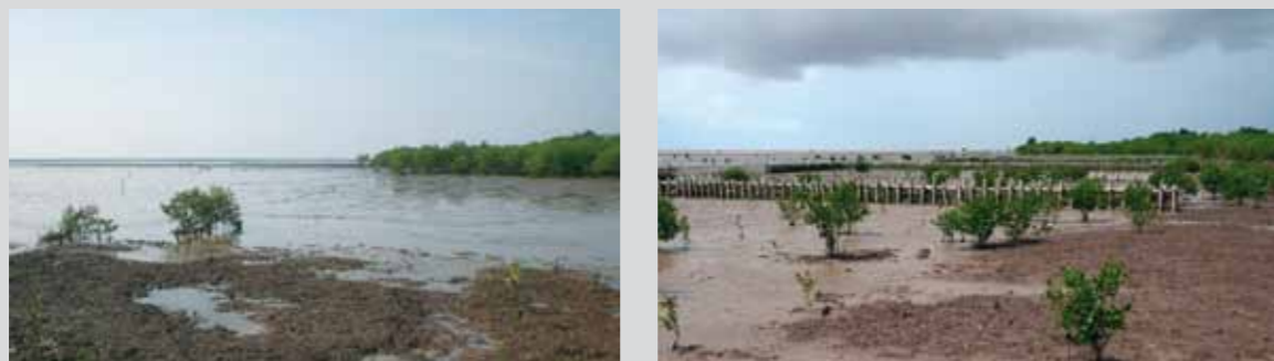
Figure 50: Changes at site 4 at the coast of Bac Lieu Province after installation of the T-shaped bamboo fences, photos from May 2012 (left), September 2012 (middle) and December 2012 (right); (Photos: Steurer)
