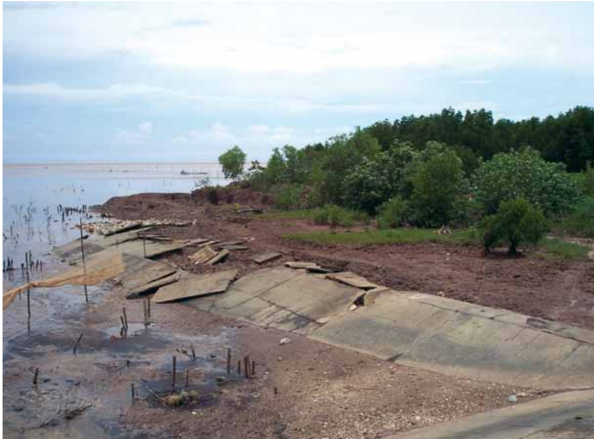
Figure 33: Damaged revetment at sluice gate 2 in Soc Trang Province; (Photo: Albers)
