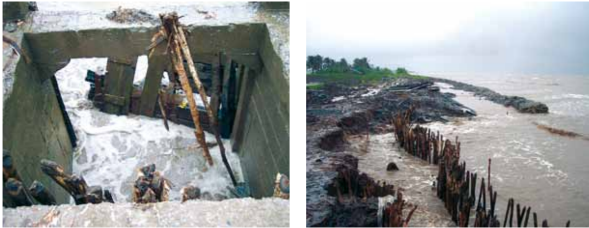
Figure 56: Damaged sluice gate (left) and erosion of the surrounding coastal section (right) in U Minh District in Ca Mau Province (Photos: Albers)
