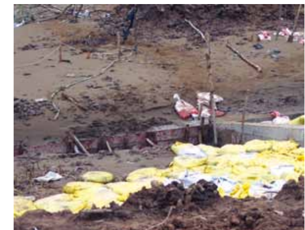
Figure 32: Revetment under construction in Soc Trang Province; different layers (left) and construction of the toe protection (right); (Photos: Albers)
