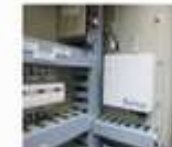
Remote monitoring equipment
